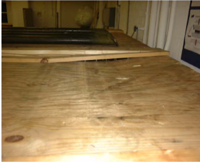
Fig. 9: Top of detector crate damaged (outside view)
