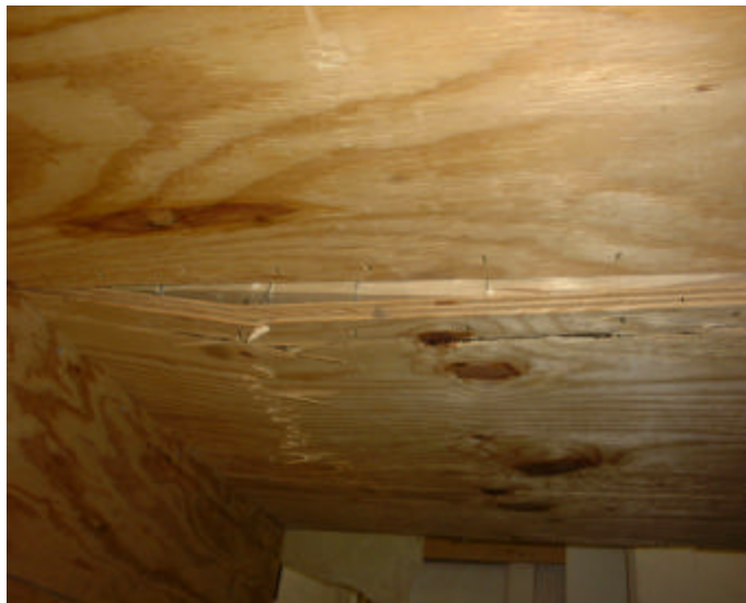
Fig. 10: Top of detector crate damaged (inside view)
